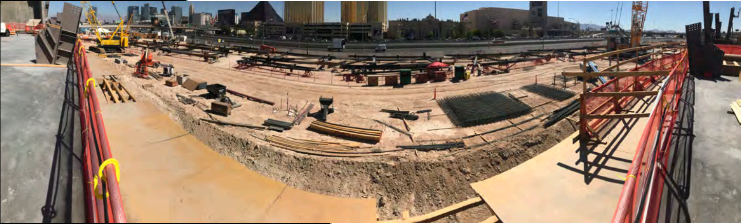
Panorama view looking east toward the Strip from the Main Concourse. Steel truss assembly taking place prior to erection.
